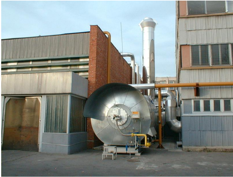
Figure 1 WK TNV 65 reheating equipment in Alföldi Printing House
